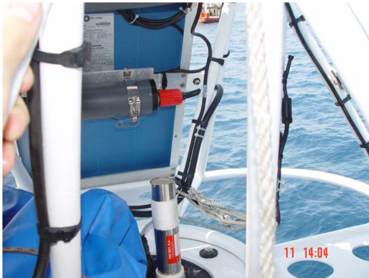
Fig 1. A MICREL ® inclinometer has been installed in the head of the buoy inner space, as the DACNet inclinometer was suspected to be out of order.
