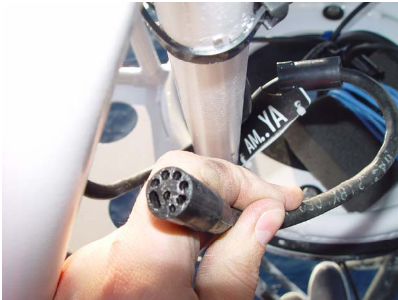
Fig 1. Damaged “DACNet to CISCO” cable.
